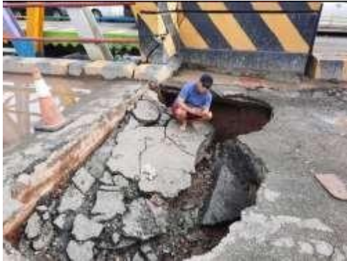
Figure 1. The sinkhole that occurred on the oprit bridge.
