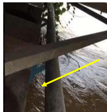
Figure 4. The heavy current that occurs under the bridge abutment.
