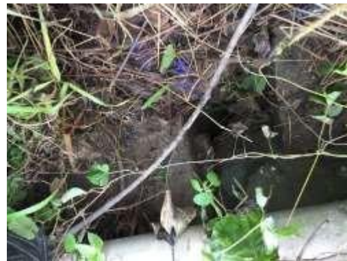
Figure 3. Gap behind the bridge abutment.
