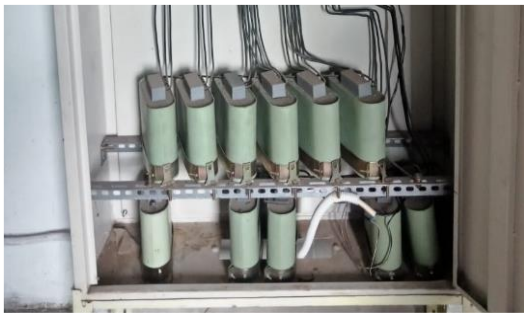
Gambar 6. Instalasi panel kapasitor bank
